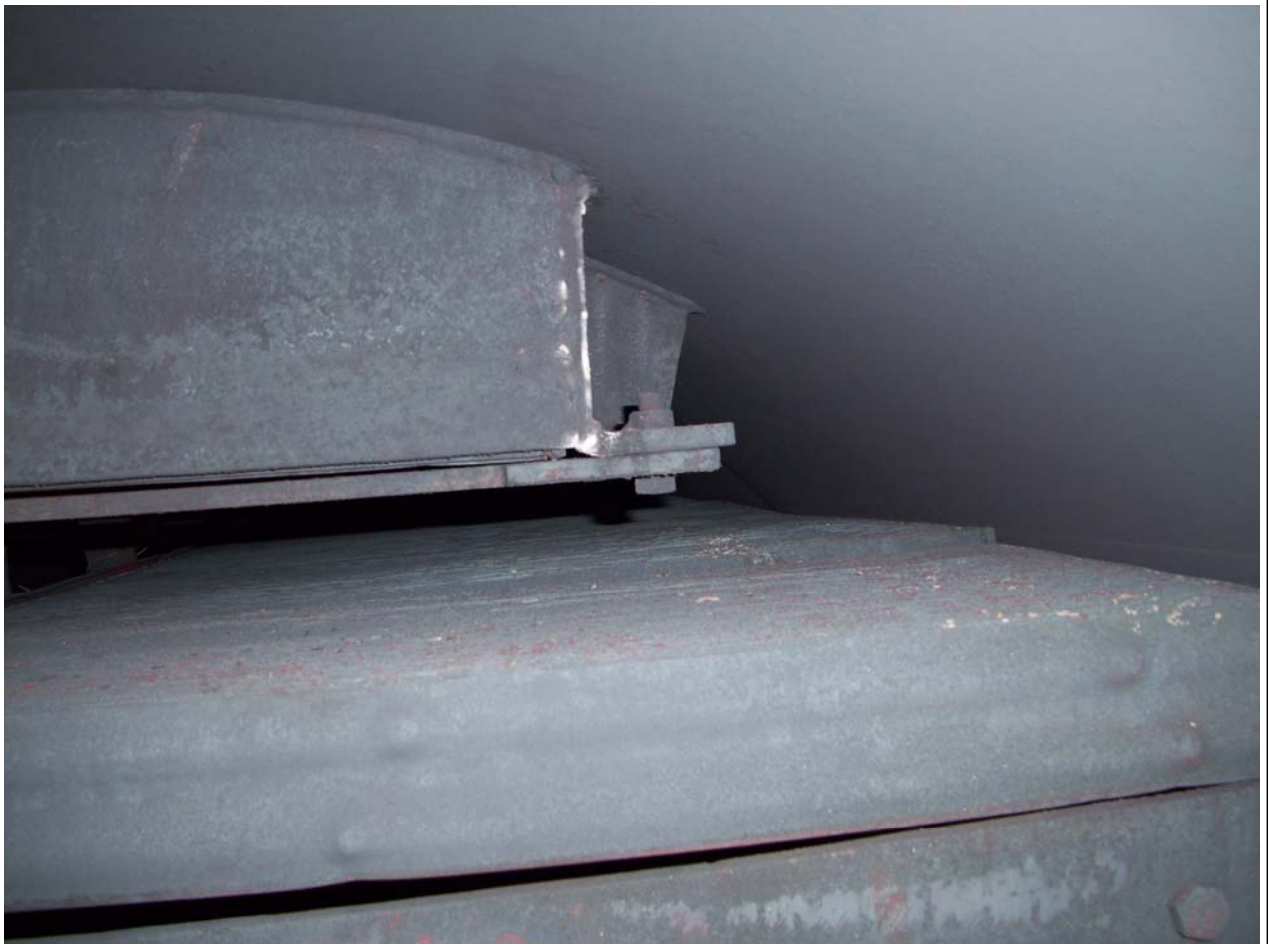
Photo 3: Presence of whitish deposit in the second stage drier.
