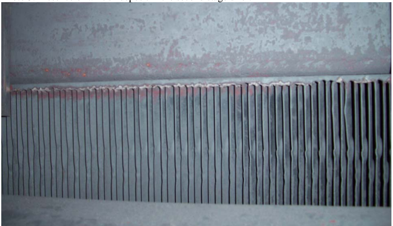
Photo 4: The presence of whitish marks along the edge of the primary drier in the steam space.
