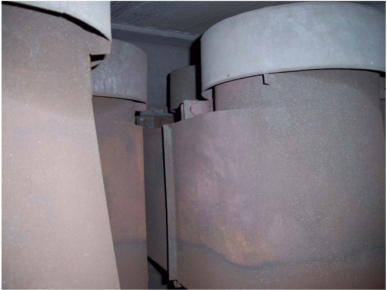
Photo 5: The whitish sparkling particles seen above the normal water level in the drum. This must be due to foaming created by excess phosphate chemical dosing in the drum. The dosing had been on when the boiler was under slumped condition.
