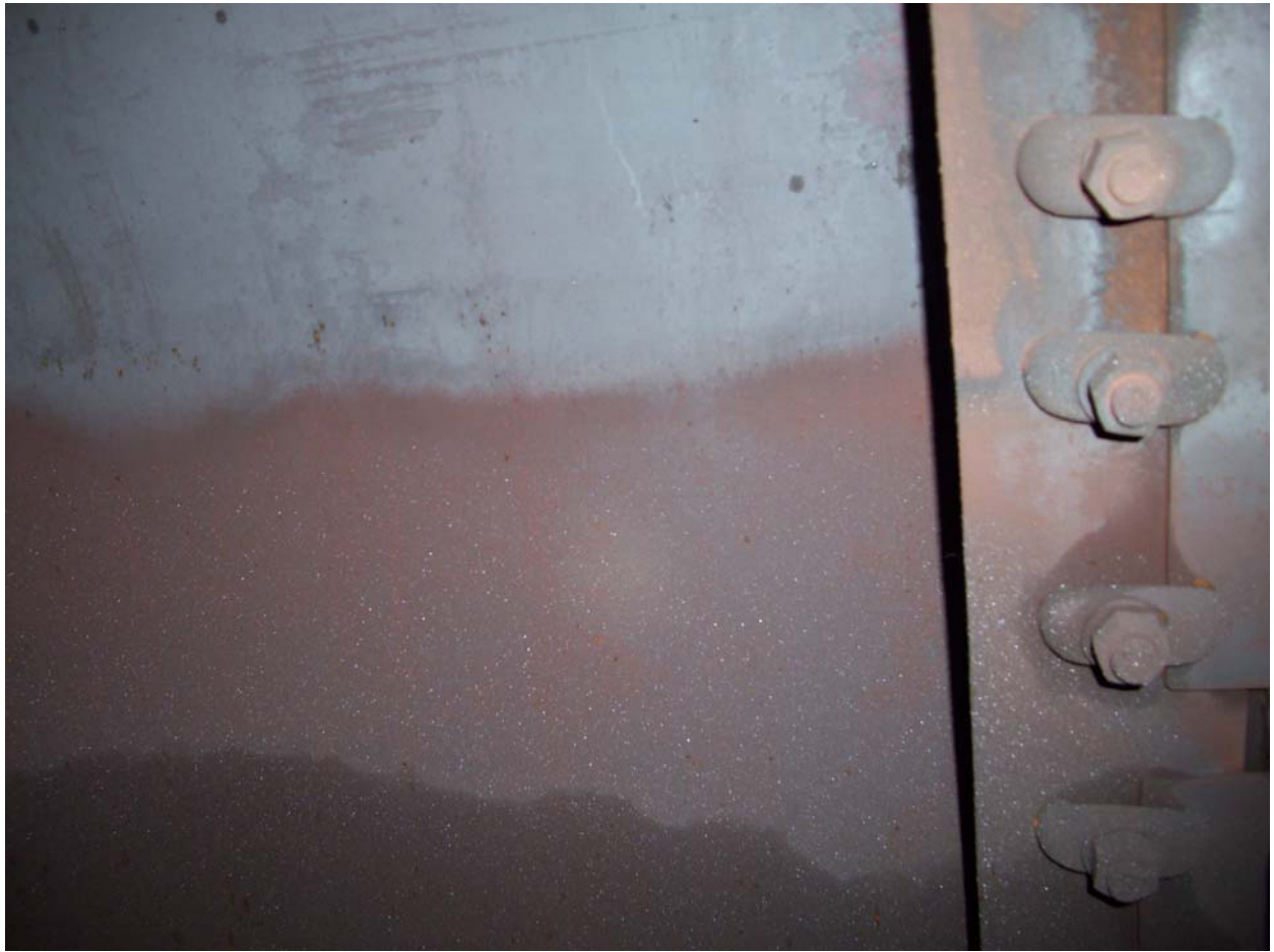
Photo 7: The boiler water chemistry had not been alright. The boiler water regime had been outside the even the coordinated phosphate control curve.
