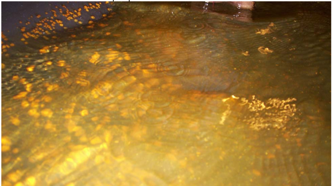
Photo 10: Presence of mud in the boiler water. The back filling of SH to be practiced to avoid carryover of dirt to SH sections.
