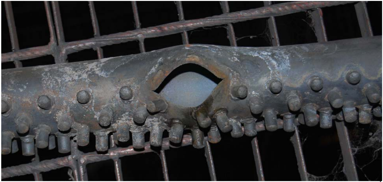
Photo 1: This is the bed SH tube failure experienced. The failed portion is in the 3 rd compartment. The edge of the failed portion of the tube is thin in nature. This indicates there has been sudden overheating situation.
